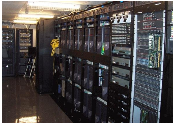
Computer racks housing the Williamson County PMBO
